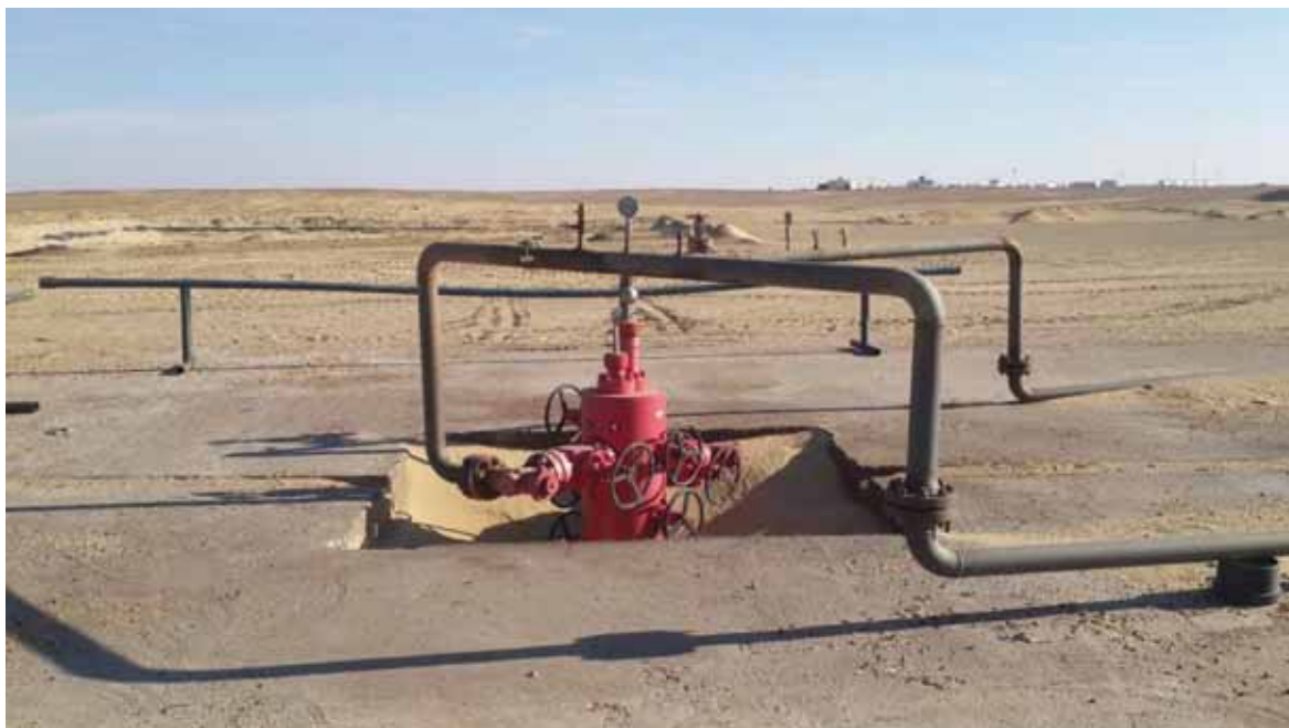
Figure AIII.18: El Salmiya – 6 Well
