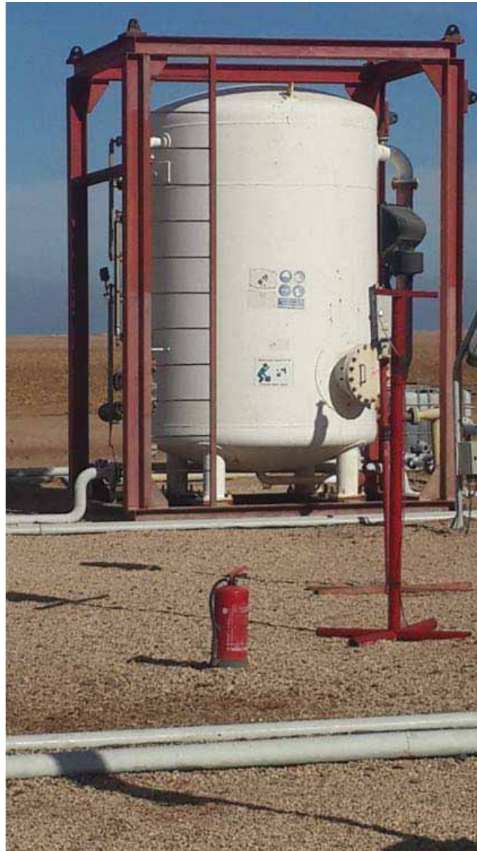
Figure AIII.20: Gas Scrubber
