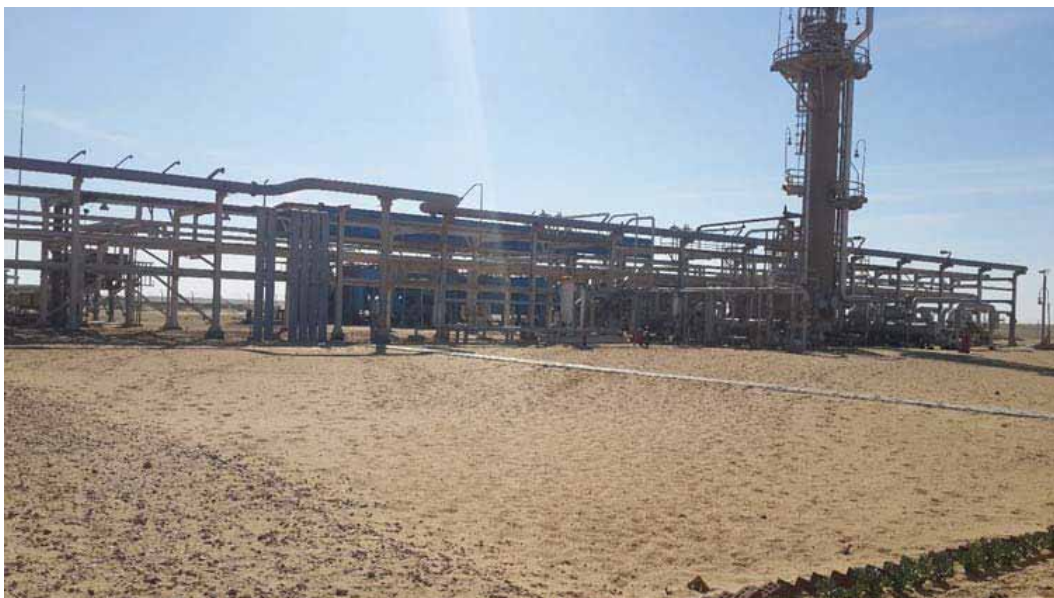
Figure AIII.14: General View of Gas Facility
