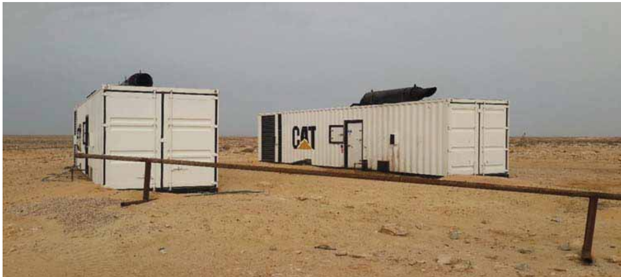
Figure AIII.6: CAT Generators
