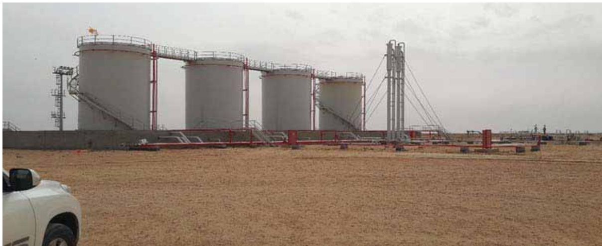
Figure AIII.1: Storage Tanks
