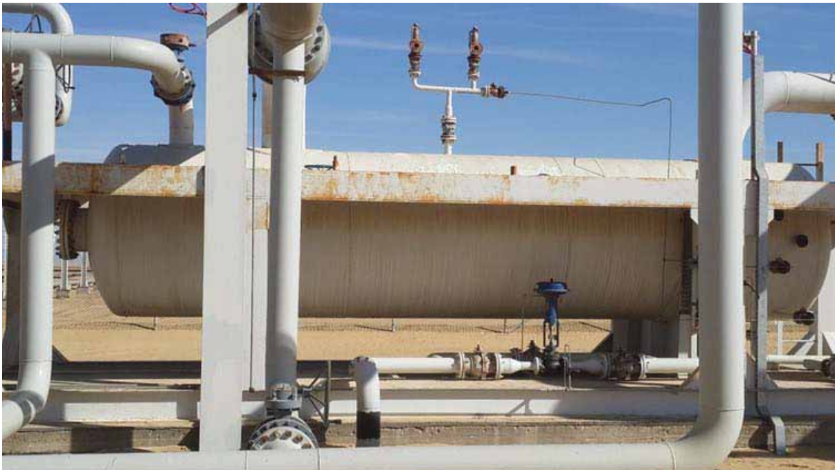
Figure AIII.15: FWKO Vessel and its Valves
