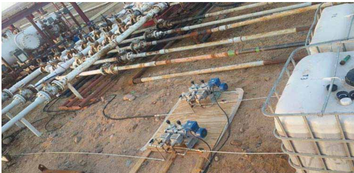
Figure AIII.22: Manifolds and Flowline Condition
