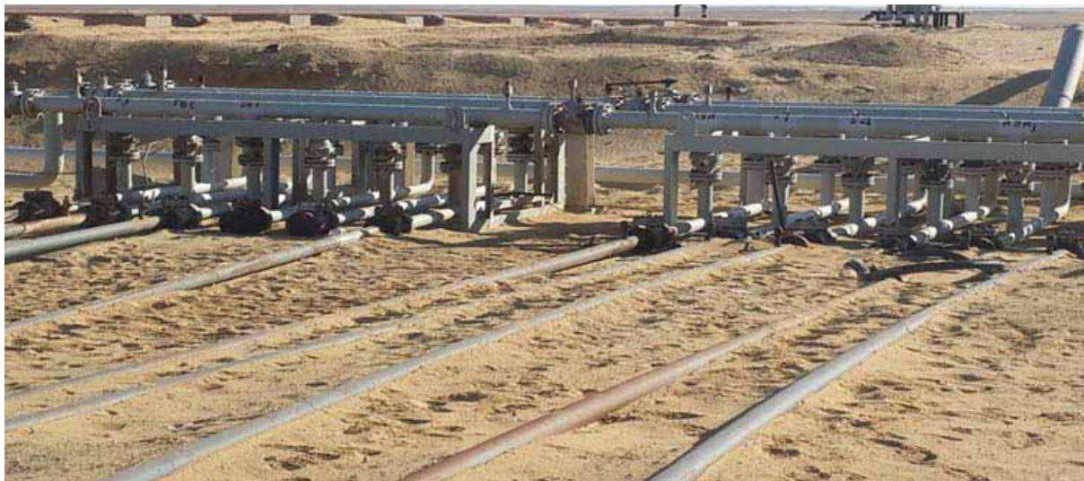
Figure AIII.11: Production Manifold at El Salmiya Oil Station
