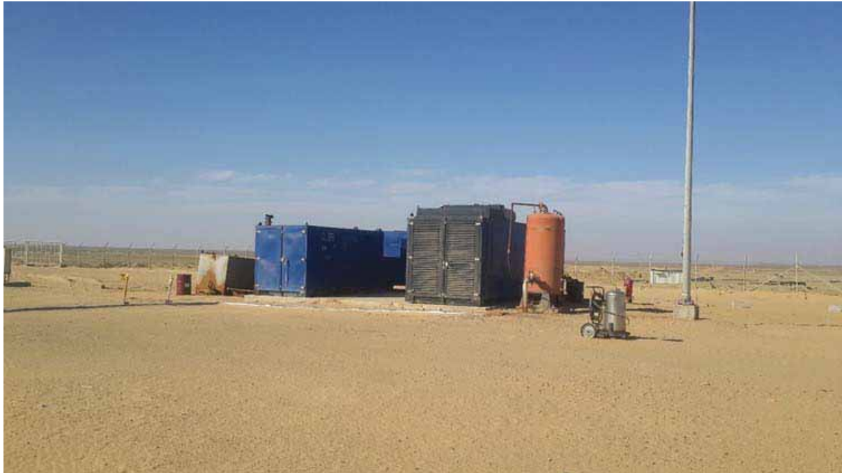
Figure AIII.16: Power Generators
