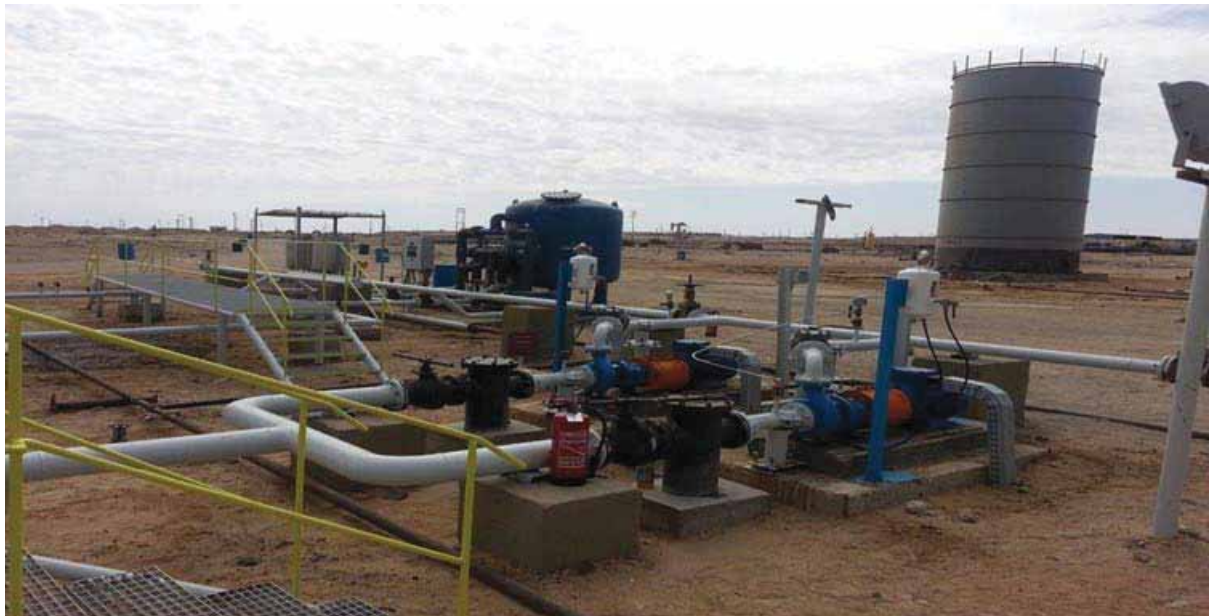
Figure AIII.26: Oil Shipping Pumps inside SHNW Station
