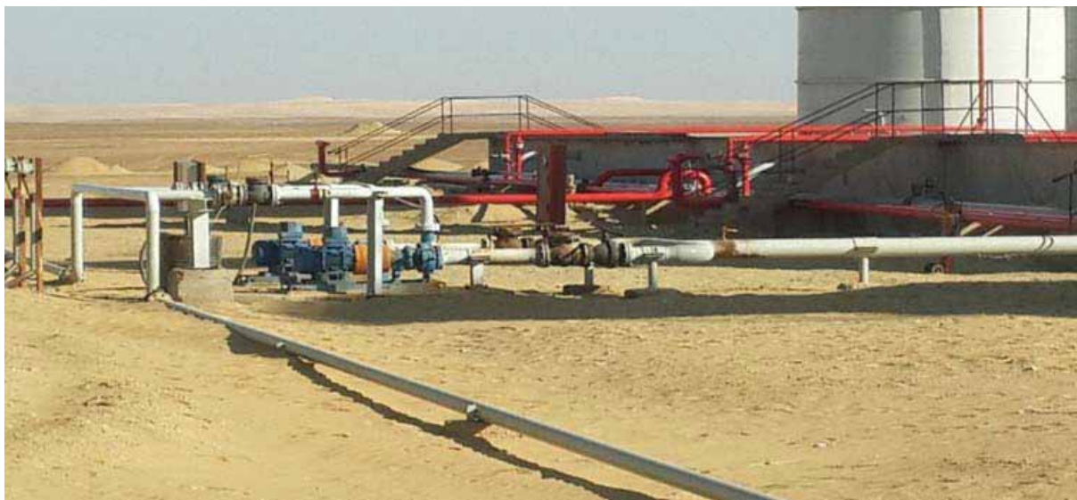
Figure AIII.13: Shipping Pumps at El Salmiya Oil Station
