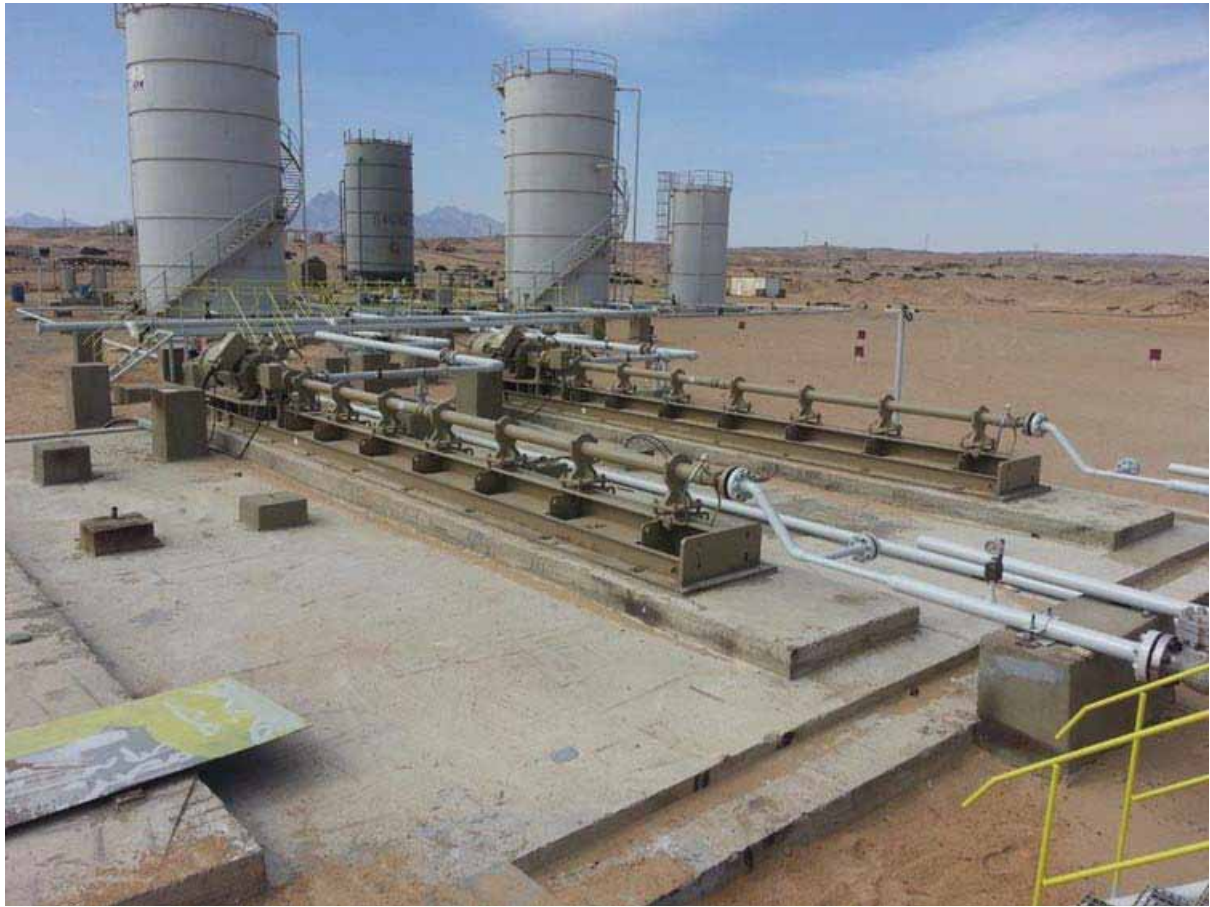
Figure AIII.25: Yusr Water Flood Facilities
