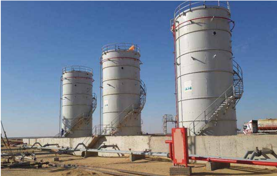
Figure AIII.10: Production Tanks at El Salmiya Oil Station
