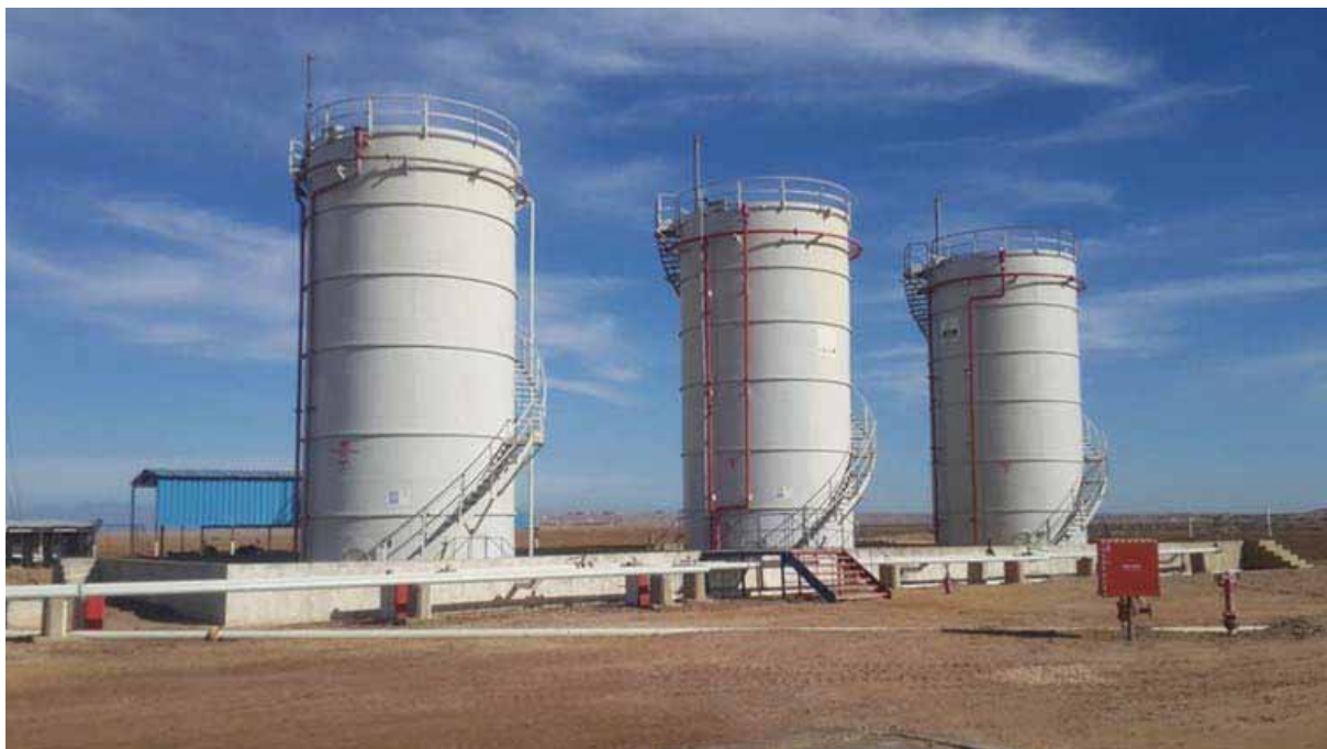
Figure AIII.19: SHNW Storage Tanks
